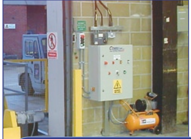
Electrical control cabinet and pneumatic services installed by our own engineers.
