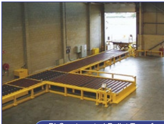
PLC automated Pallet Transfer
